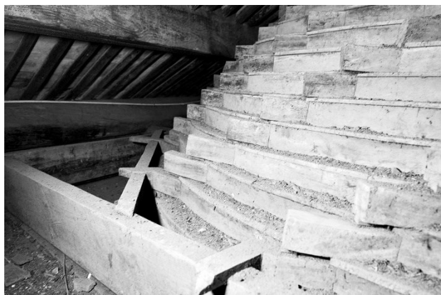
Figure 6. Space between the upper roof structure and the spiral zaojing. Ref. ZJ-01, built in the 1920s, in Ninghai.
