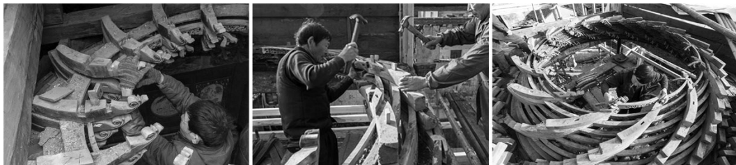
Figure 9. Renovation of the spiral zaojing in Family Ye's ancestral temple, 2016. Left, dismant of the 18th layer. Middle, hammering of the reassembled zaojing. Right, close to completion. Photo: Xiaodong Chai.
