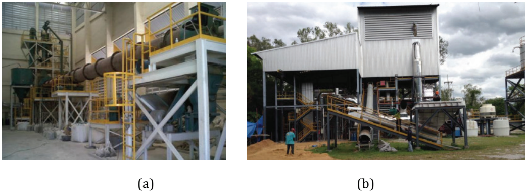
Figure 5.1 Pilot scale production for clay calcination (a) Rotary kiln (b) Fluidized bed
