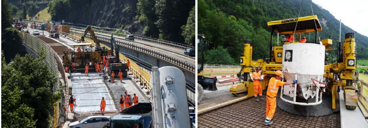
Figure 10. General view of construction site on 12 th of July 2018 (left; Photo A.Wey keystone), and UHPFRC casting using a finisher (right).
