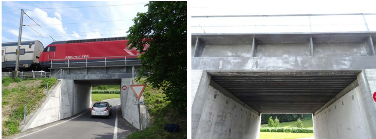
Figure 15. Railway underpass Unterwalden with a structure in R-UHPFRC resting on concrete abutments (left); edge girder and ribbed plate girder of the structure in reinforced UHPFRC.
