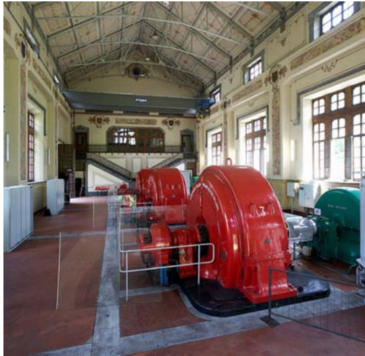
Fig. 4. Picture of the Champagne 1 hydropower plant (source: Compagnia Valdostana delle Acque)
