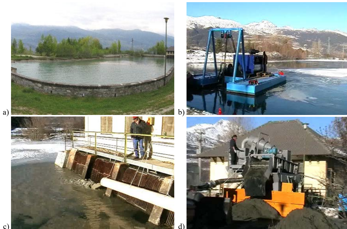
Fig. 5. a) View of the Sorressamont accumulation basin (source: ARPA Valle d'Aosta), b) installation in 2006 of the floating modular unit, c) the introduction of the fine sediments into the water intake and d) the on-shore sediment treatment plant
