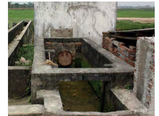
Figure 28 Station de pompage Can Co (irrigation et drainage)
