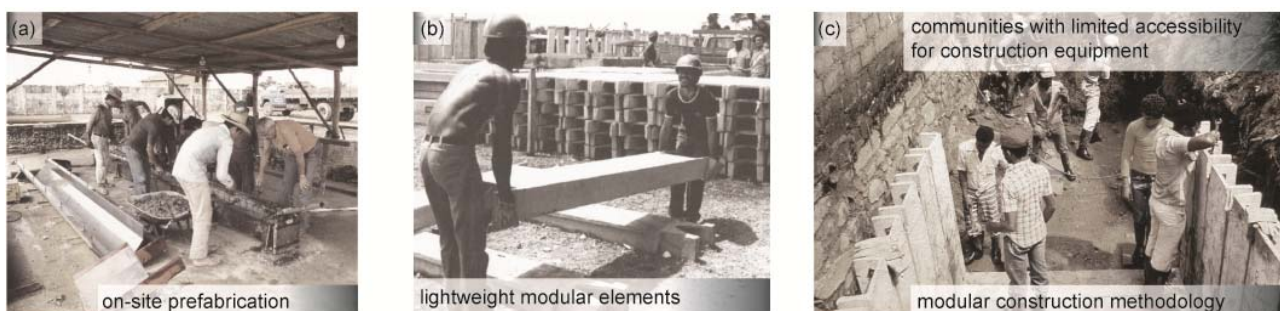
Figure 3. Lelé's flexible construction system with lightweight ferrocement elements: (a) on-site miniplant [1,pp 141]; (b) transportability of elements [1,pp 106]; (c) assembly within hardly accessible area (favela) [1,pp 106].
