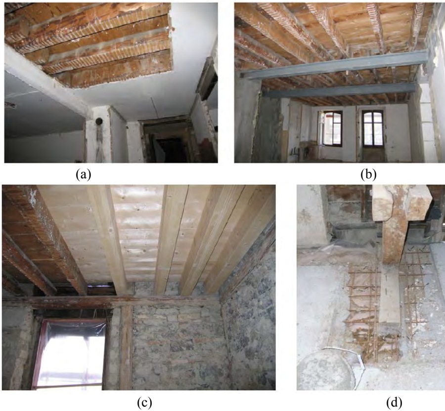
Figure 3. Retrofit of the slabs in the building (a) initial state, (b) added steel beams, (c) renewal of the wooden floors, and (d) added RC slabs
