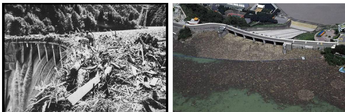
Figure 1 Picture of Palagnedra dam (left) (Bruschin, Bauer, Delley, & Trucco, 1982) and Shihmen Reservoir (right) (Chen & Chao, 2010).
