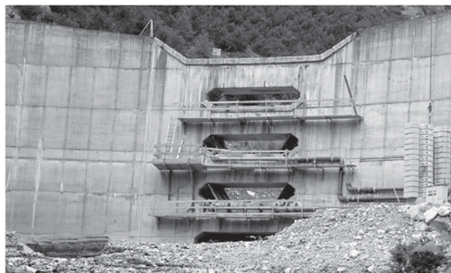
Fig. 15. Picture of the slot barrier at the Schnannerbach torrent (Austria) after the flood event in August 2005; view from downstream (source: Michael Sturm, Uni Innsbruck, with permission).
