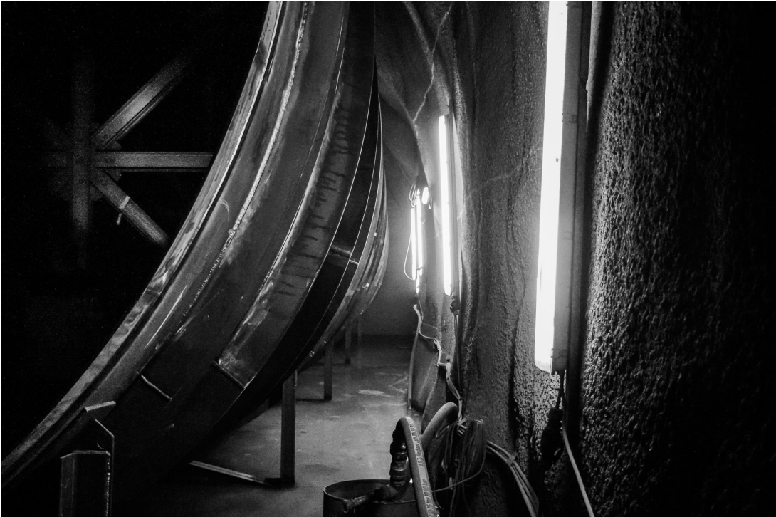
(f) Void between the steel liner and the surrounding rock (with shotcrete), before backfilling with concrete.
