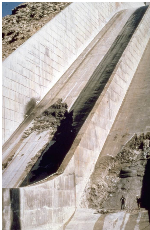
Figure 1.1 – Cavitation damages on the Karun dam spillway 1987 (photo: Prof. Hans-Erwin Minor)
