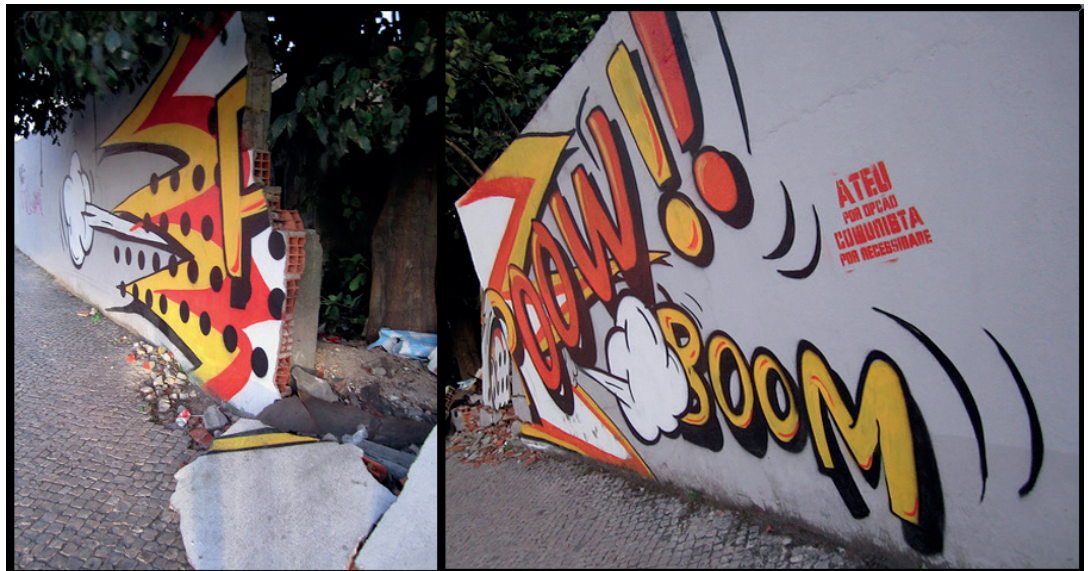
Img 56. Broken wall in Campo de Ourique, and a painting of a cartoon-style explosion. This painting was later replaced by a publicity mural.
