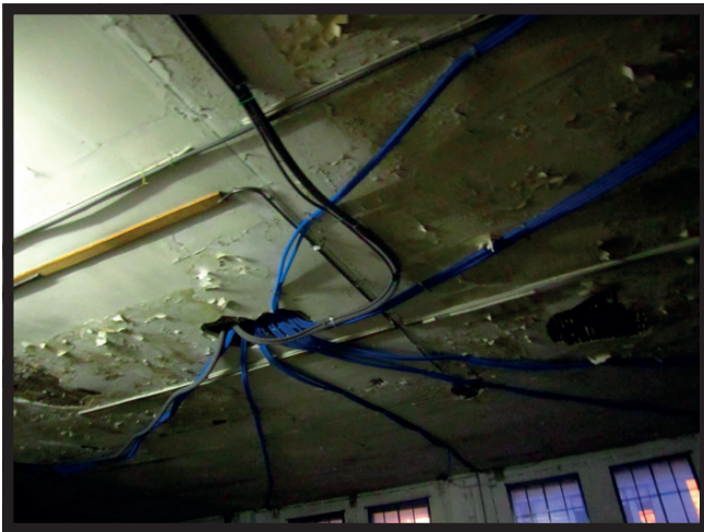
Img 335. DIY adaptations to the needs of the users: wires and pipes along walls and ceilings.
