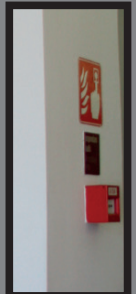
Img 254. Surveillance cameras and fire extinguishers and alarms.
