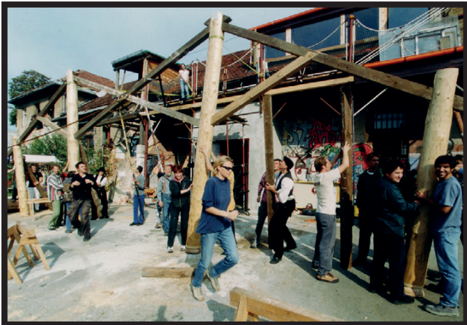
Img 244. The curious roof of Menza pri Koritu, made by Axt und Kelle (ource: Kud Mreza 2001)
