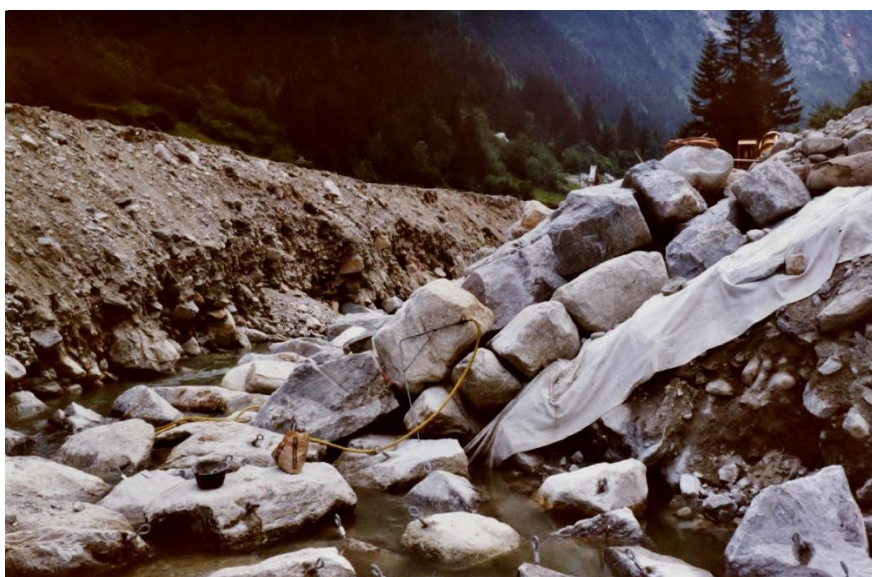
Figure 6.1 Riprap built of individually placed large blocks in two layers on Reuss river in Switzerland (by A.J. Schleiss, 1988)
