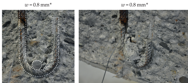
Figure 3.20 Saw-cut performed after test in specimen SB14 with deformed hooks disposed parallel to cracks with long bar (dashed line for initial position and geometry of the detail)
