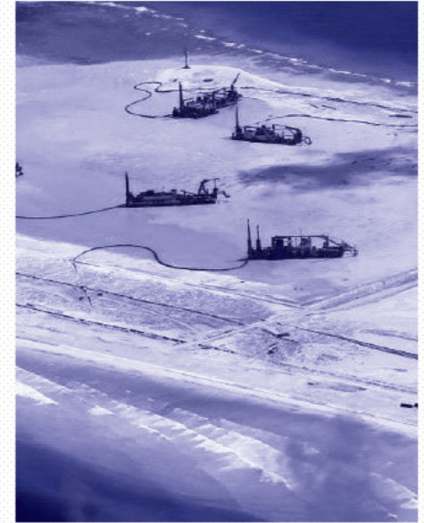
Fig. 13 : Picture of the artificial island under construction in the South China Sea by the Chinese army, 2015. The Guardian
