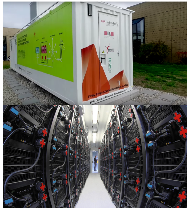
Fig. 7. An outside (top picture) and inside view (bottom picture) of the 720 kVA/500 kWh Lithium Titanate-based BESS used in this experimental work. The system, developed by Leclanché, includes a four-quadrant fully controllable DC/AC converter and a 0.3/20 kV step-up transformer. It is hosted in a temperature controlled container (picture of Alain Herzog, EPFL).
