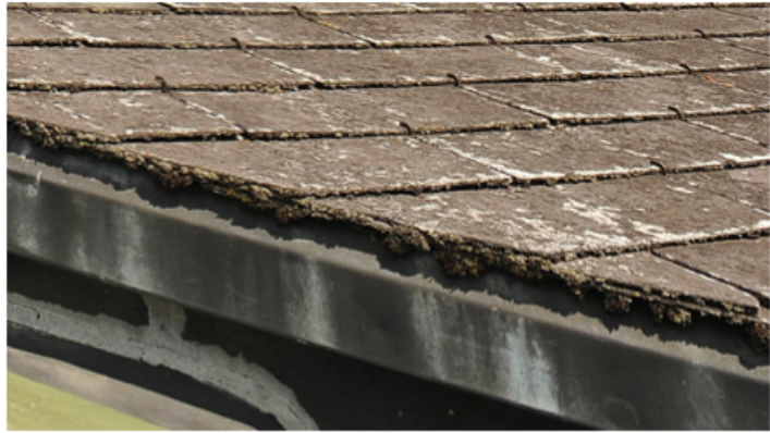
Figure 5.2-17: A closer look of the weather beaten roof tiles. (Photo credit: Christian Röske)
