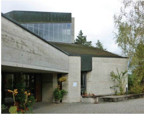
Figure 5.2-16: The roof quality of the church from afar. It can be seen from the greenish colour that mosses fully occupy the roof tiles today.
