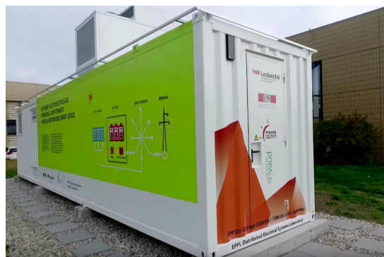
Fig. 1. The 720kVA/500 kWh grid-connected BESS installed at the Swiss Federal Institute of Technology of Lausanne (EPFL) used to validate the “dispatchable feeder” concept.
