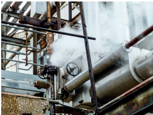
(c) Leaky valve.
