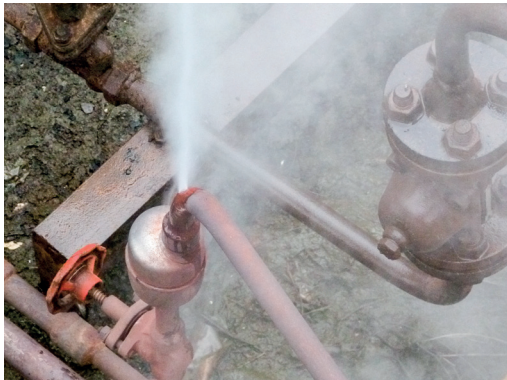
(a) Ruptured pipe.
