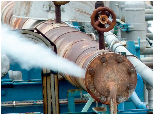
(b) Leaky seal.
