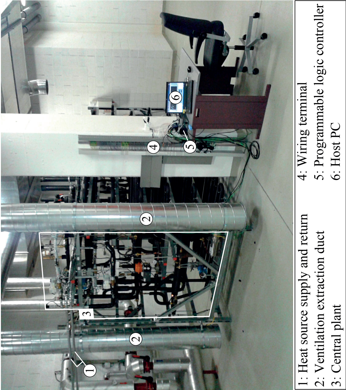
Figure 2.2 – View of the test facility on the central plant side.
