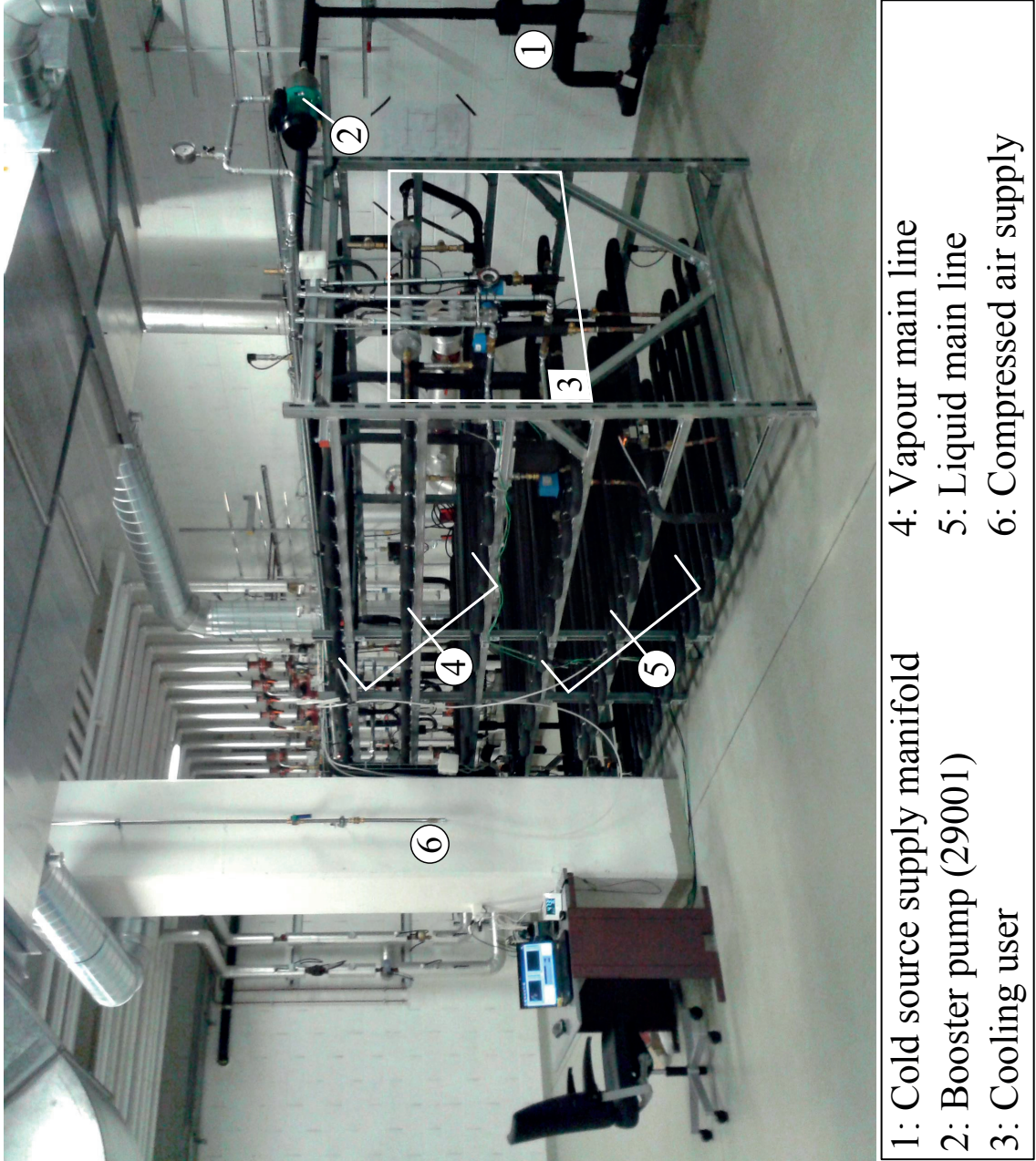
Figure 2.3 – View of the test facility on the cooling user side.
