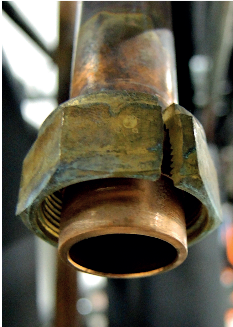
Figure 2.25 – Close view of the bolt of the fitting that burst, causing a large leak of CO 2 that triggered both the gas detection and the pressure switch safety chains.
