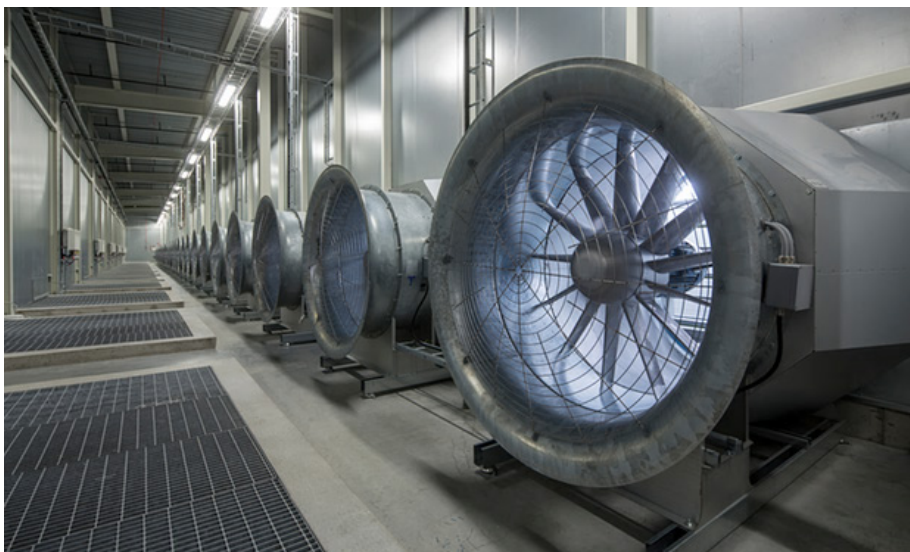
The Facebook data centre in northern Sweden. Photograph: David Levene for the Guardian, Source: www.theguardian.com
