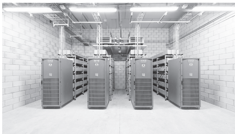
Figure 1.3 The Internet machine film documents the usually invisible infrastructures of the Internet in a data center in Alcalá, Spain. It features server racks, routers, cables, corridors, relays and power generators, and transmits some of the noise and energy that exist around this infrastructure. A still from the film by Timo Arnall
