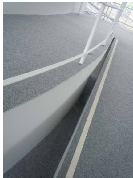
Photo 211. The folds in the wheel chair ramps do not afford the use of ordinary equipment like vacuum cleaners. June 2012.
