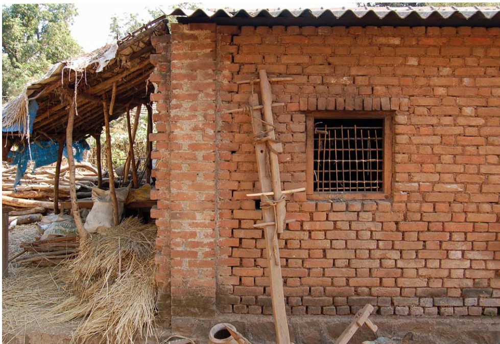
Photo 24. The use of cement mortar in this corner column is a handshake of pucca and kacca . The wall is made of earth mortar masonry and affords easy future changes while keeping the main structure. The indentations on the left are a provision for future extension. Near Vasind, February 27, 2010.
