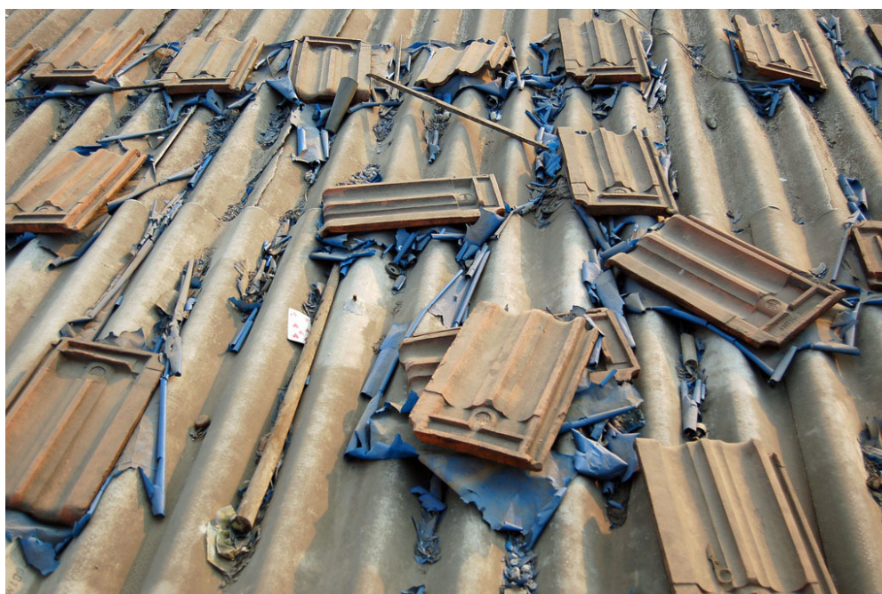
Photo 112. Blue tarpaulins however disintegrate under sunlight. January 25, 2010.
