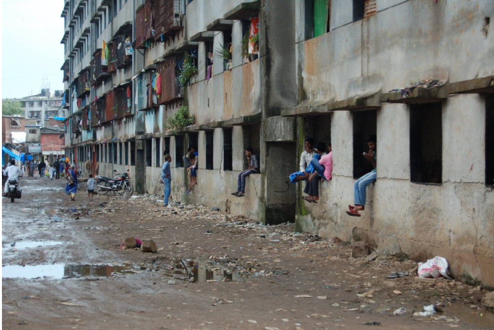
Photo 200. Kolya Khata's ground floor has become a hangout for glue sniffers and drug addicts. Kuttiwadi, July 25, 2014.
