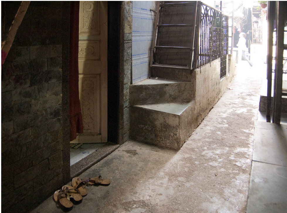
Photo 109. Raised floor levels show results of negotiation. The concrete steps making a turn allow the stairs to come down without landing too much on the neighbor's doorstep. Future redevelopment of the house on the left and its subsequent steps will not hinder the existing. January 17, 2013.
