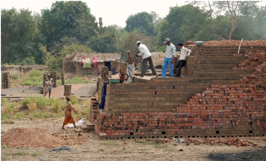
Photo 31. Building a new kiln stack. The firing process changes the color of the bricks from green to red. Insufficiently fired bricks are reused in the skin of kiln. Near Vasind, February 10, 2010.
