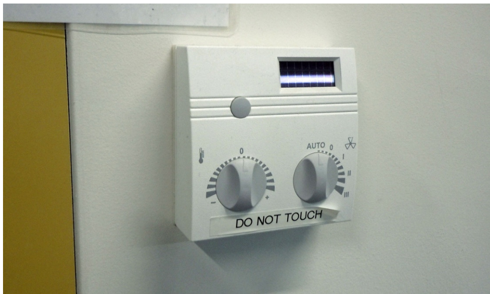
Photo 10. The autonomy of its occupants overloaded the climate system in this office building, hence the heteronomous intervention. Rolle, CH April 18, 2012.
