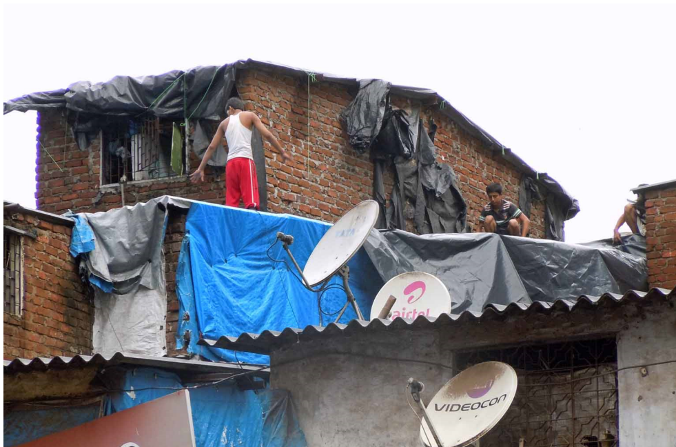
Photo 123. A familiar sight in early monsoon: men fitting plastic sheet over an asbestos-cement roof in Dharavi. July 11, 2014.
