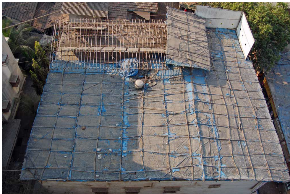
Photo 111. Blue tarpaulins fixed on top of asbestos cement sheets, in order to improve water tightness. January 26, 2010.
