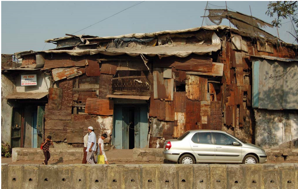
Photo 46. Sheets of corrugated steel used here in a non-repetitive and non-systemic way. January 15, 2009.
