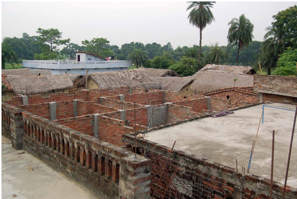
Photo 121. Modernization in Susant village in Bihar. Concrete columns and slabs replace the traditional pitched roofs of wood and rice thatch. August 2, 2014.
