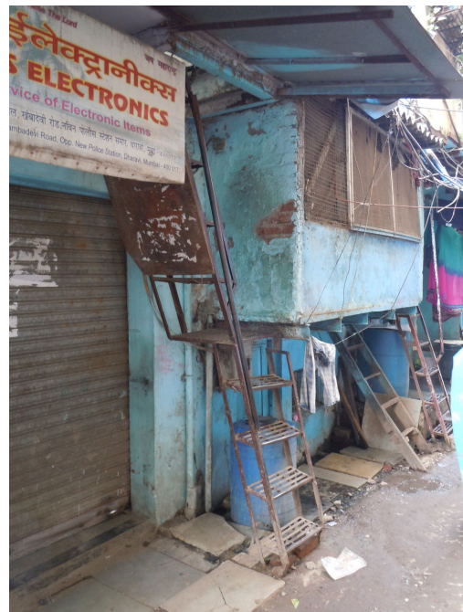
Photo 105. Street level reaches halfway the ground floor story. January 21, 2013.
