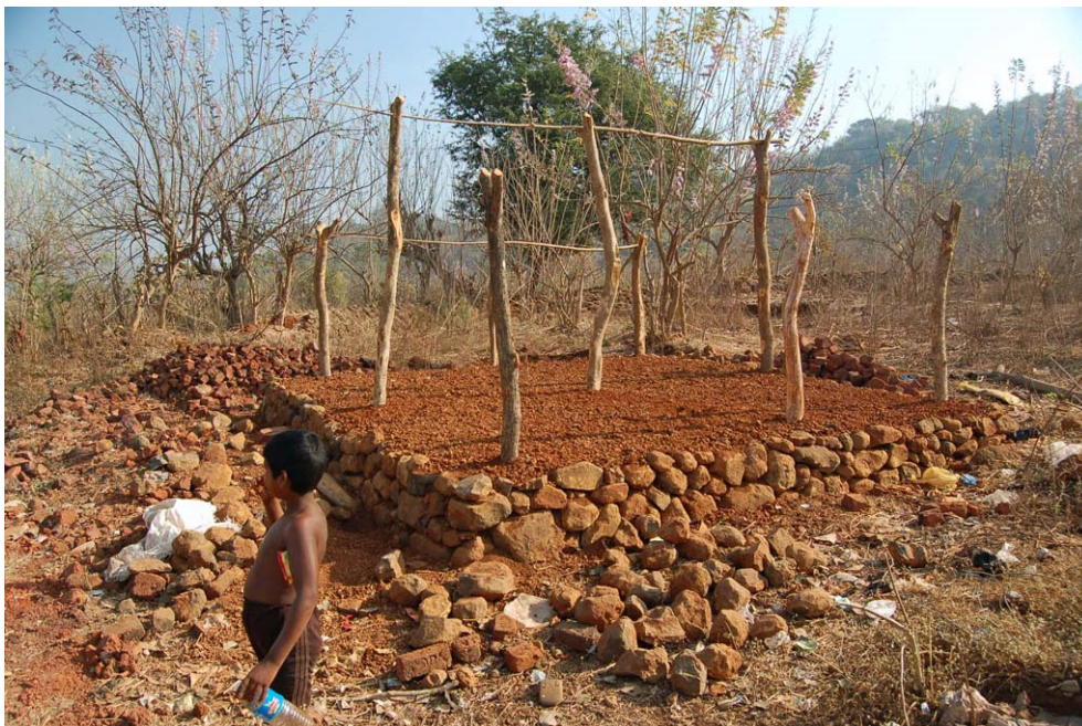
Photo 22. Base and beginning of a wooden structure for a kacca house. All materials come from the site's immediate vicinity. A dry wall, i.e. without mortar or cement, surrounds the base. Tara, February 18, 2010.
