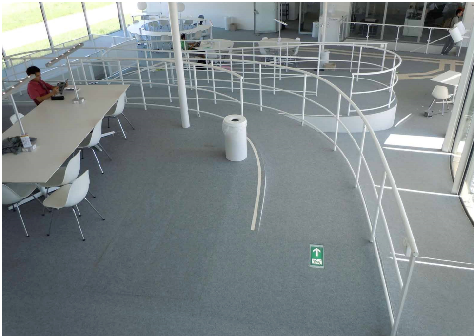
Photo 214. Wheelchair ramp folded into hairpin bends. The floor along the windows on the right is too steep for a legally acceptable escape route, hence the indicator in the floor recommending the zigzag route. June 2012.
