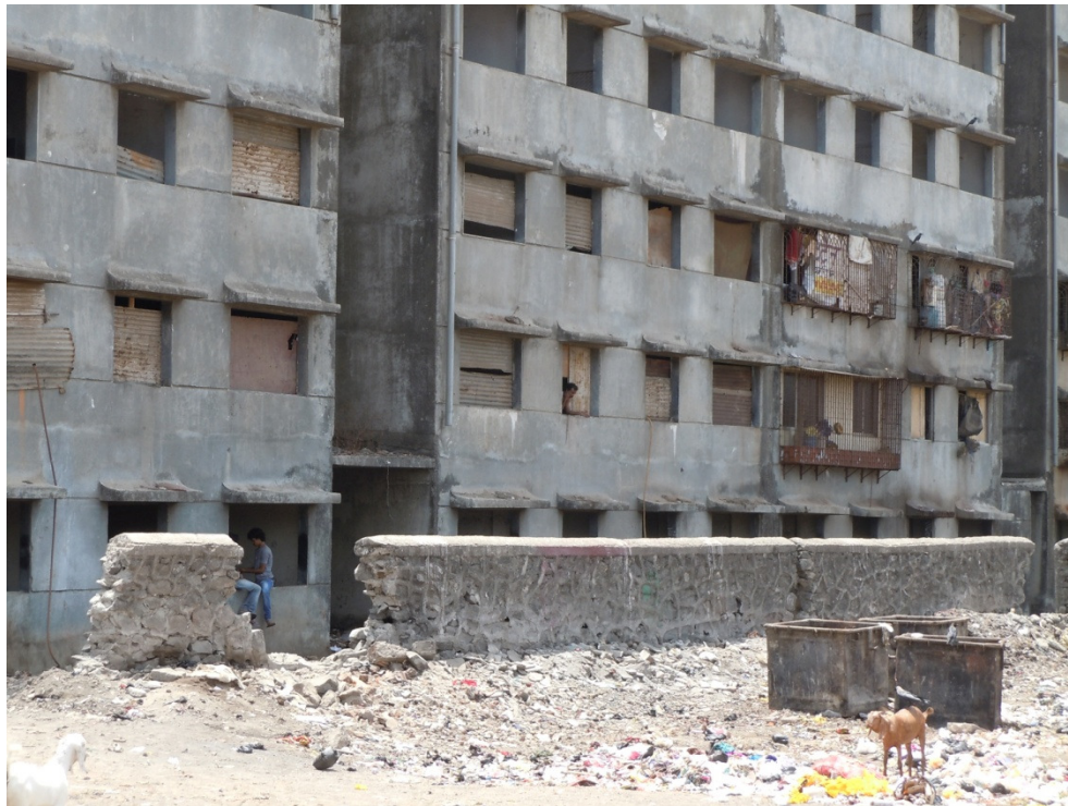
Photo 183. Kolya Khata is a failed product of the formal sector. Since utilities and services are missing, squatters have only encroached on the first and second floor. The informal sector cannot handle the rest of the building. April 19, 2013.
