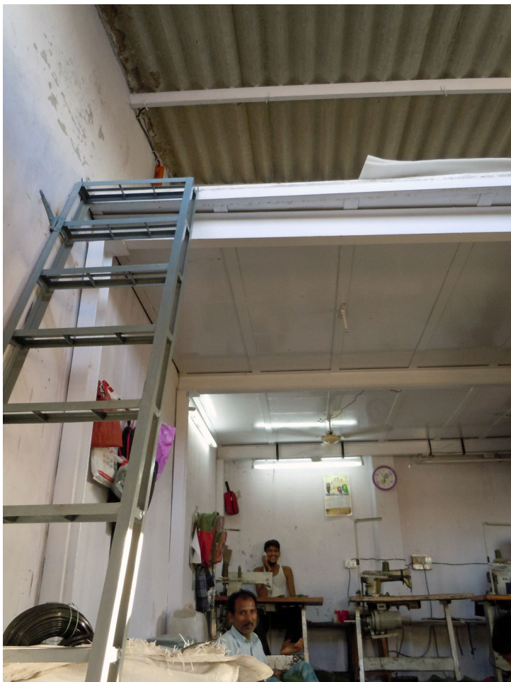
Photo 118. A mezzanine floor in a workshop blocks heat radiation and provides storage space. Dharavi, April 8, 2013.
