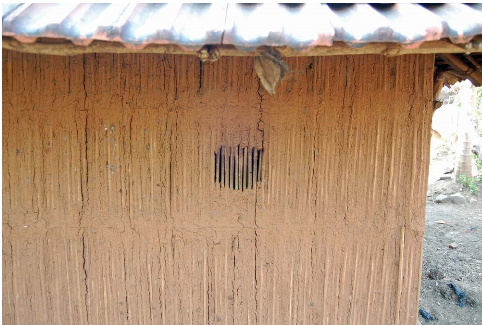
Photo 26. It is easy to create a ventilation grill in a kacca wall. Kelthan, January 18, 2013.
