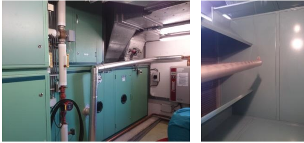
Figure 3. Air Handling Unit and steam pipe
