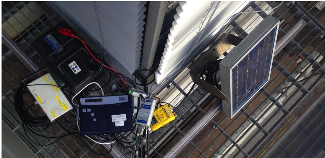
Figure 1: Equipment installed in the DSF to power anemometers to monitor air flow in DSF.
