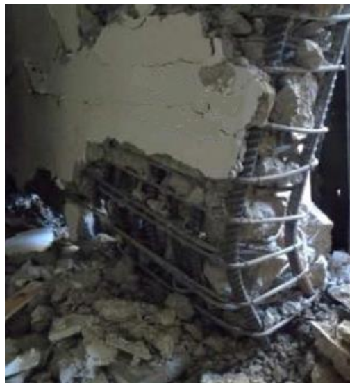
Fig. 1 Example of out-of-plane induced damage in a RC wall after the New Zealand earthquake (Sritharan et al. 2014).
