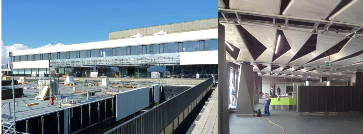
Figure 2: Exterior view of CHUV installation (left); Indoor view at the end of the first step of the installation (right).
