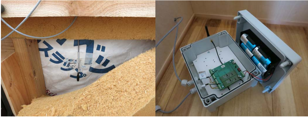
Figure 4: The installation of sensors. (left: an sensor inserted between air-tight membrane and insulation, right: a sensor node box)
