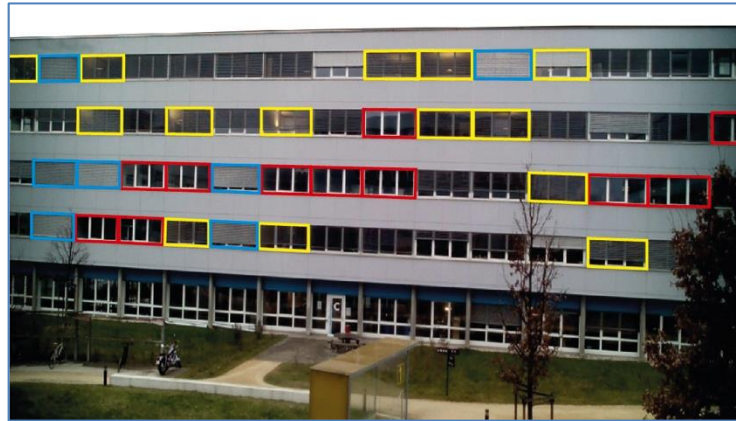
Figure 1: Photo of the west façade of building PSE-C on February 5, 2013, overcast sky
