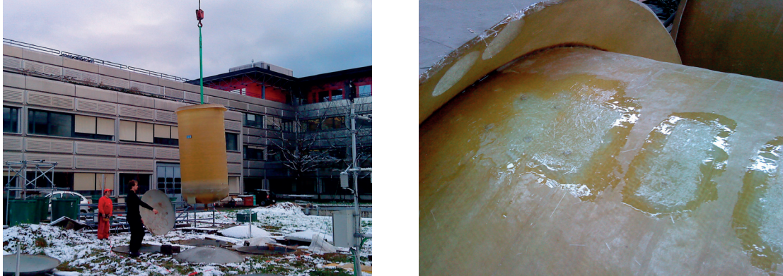
Figure A.1: Replacement of the lysimeter tank in the compartment (left). Previous holes drilled in the wall were filled with polyester resin and reinforced with fiberglass mat (right).
