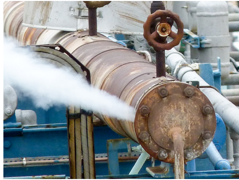
(b) Leaky seal.
