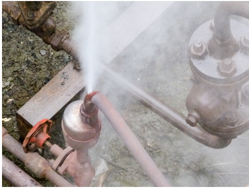
(a) Ruptured pipe.
