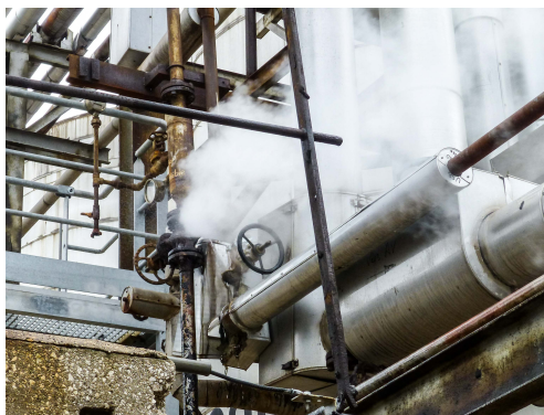
(c) Leaky valve.
