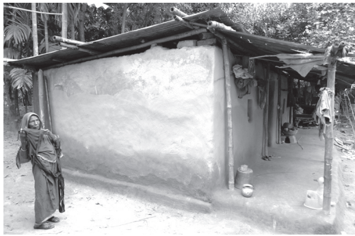
Figure 7. Raipur Village (Mymensingh region): the walls act as an independent box: if damaged, the roof is preserved, providing shelter to the people and limiting the extent and complexity of repairs. Credits: A. Caimi.
