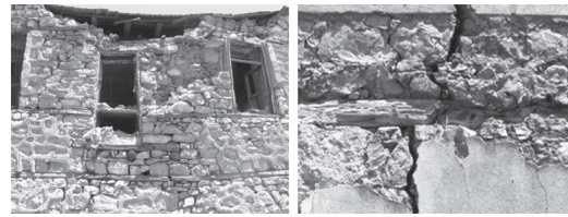
Figure 3a and 3b. Seismic damages on two different buildings in Beltchichta (Republic of Macedonia). Credits: M. Hofmann.
