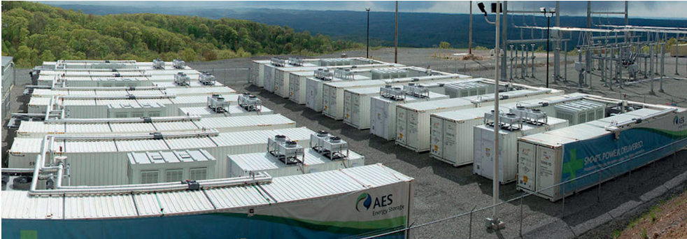
Fig. 117. 32MW/8MWh frequency regulation facility in Laurel Mountain (WV/USA) by AES Energy Storage and A123 Systems. The facility is co-operated with a 98MW wind farm.
