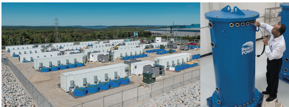
Fig. 118. 20MW/4MWh frequency regulation facility in Stephentown (NY/USA) by Beacon Power.
