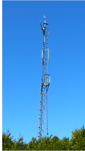
Figure 3.7: The 30 m high (effective height 26 m) Urban Climate Measurement Tower at the South East corner of the B.C. Hydro Mainwaring Substation at the Vancouver Sunset site. The tower belongs to the Micrometeorology group at UBC. Image by the author.
