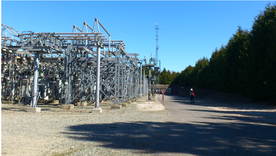
Figure 9.10: The Mainwaring Substation of B.C. Hydro in Vancouver Sunset. The UBC Research Tower is visible in the background on the right.
