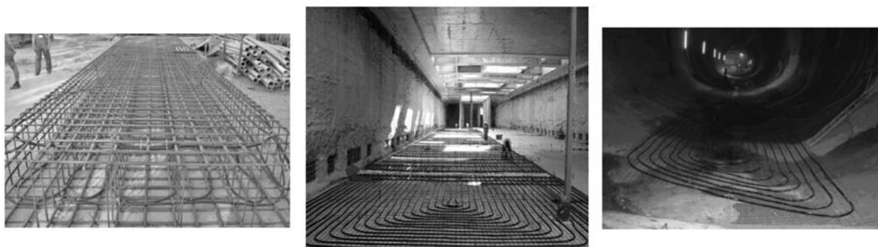
Figure 5:3 Picture of a diaphragm wall reinforcing cage equipped with absorber pipes in Vienna, Austria (left), from (Brandl, 2006), and thermoactive floor slab (middle) and tunnel invert (right), from (Adam and Markiewicz, 2009)
