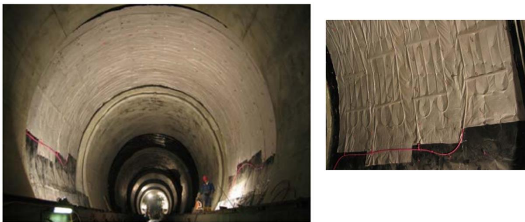
Figure 5:2 Portion of the Lainzer tunnel (Austria) equipped with thermoactive geosynthetics, from(Adam and Markiewicz, 2009)
