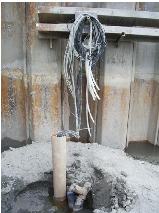
Figure 9:23 Sensor cables coming out from an instrumented pile (optical fibers in white and vibrating wires in black) through the protective PVC tube
