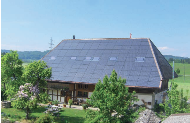
Fig. 22: Frameless c-Si full-roof BIPV installation on a 19 th century Swiss farmhouse in Uettligen (System provider: 3-S Photovoltaics, Meyer & Burger Group)
