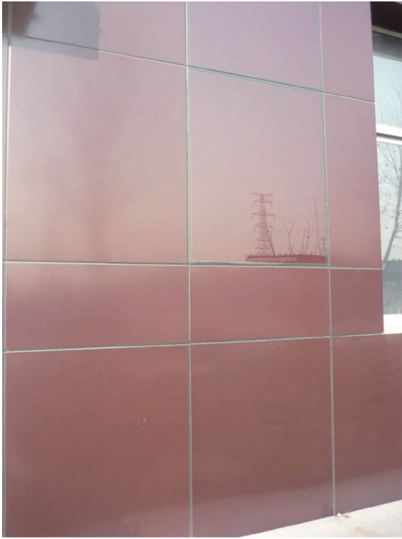
Fig. 10: Baoding (China): Detail of an a-Si façade. The active PV panel in the middle to the right is surrounded by metal façade elements of the same colour (Courtesy: Tianwei Solar Films; Photo: P. Heinsteint)
