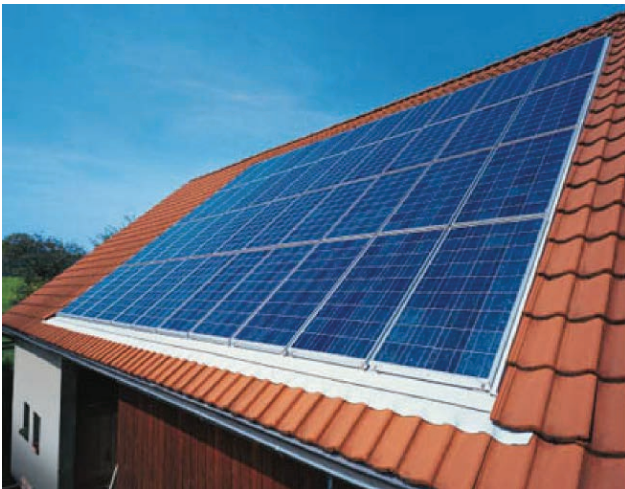
Fig. 19: Framed in-roof system: less homogenous appeal due to the contrast of the aluminium frame and the PV panels.
