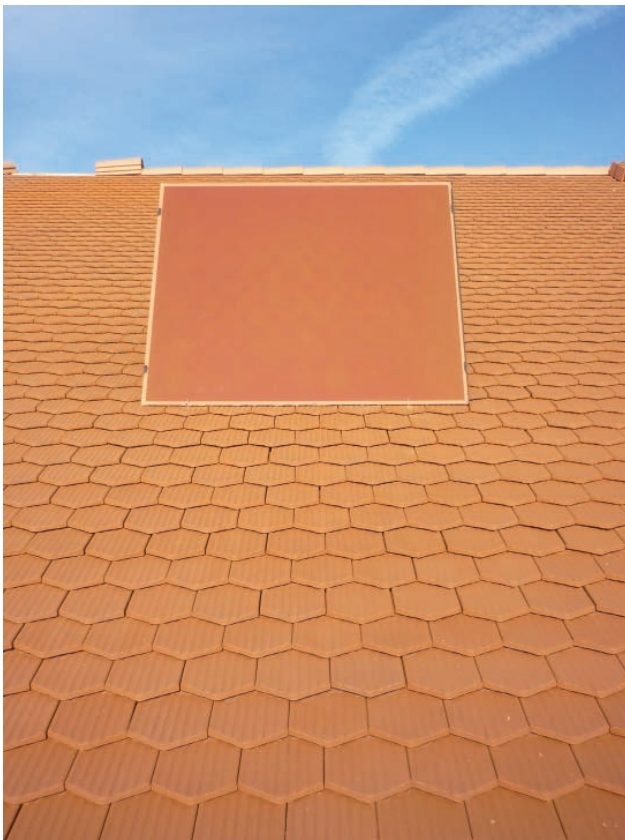
Fig. 39: Archinsolar PV module installed for testing on a traditional roof (Photo: P. Heinsteinst).
