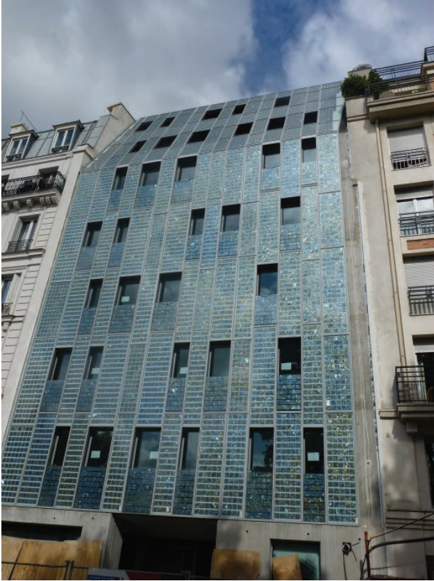
Fig. 41a: Building at Quai de Valmy 179, Paris (France): seven storey façade covered with 130 customized emerald-green multicrystalline Si panels (Surface: 173,6 m 2 ; Energy output: 17 kWp; Architects: Emmanuel Saadi and Jean-Louis Rey, System provider: Sunways AG, 2011)
