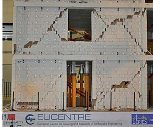
Fig. 12.16 URM walls of shake table test unit after Run 9 (Beyer et al. 2014)
