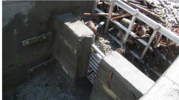
Figure 11. Situation at the dam after 100-year return period flood event on the physical model.
