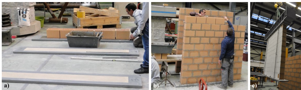
Figure 2. (a) Steel plates with layer of quartz sand, (b) test units during construction and (c) transportation of test unit to test stand
