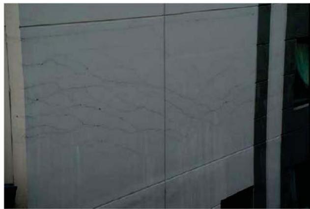
Figure 6 Well-distributed flexural cracks on a wall (Wilson and Lewis 2011)
