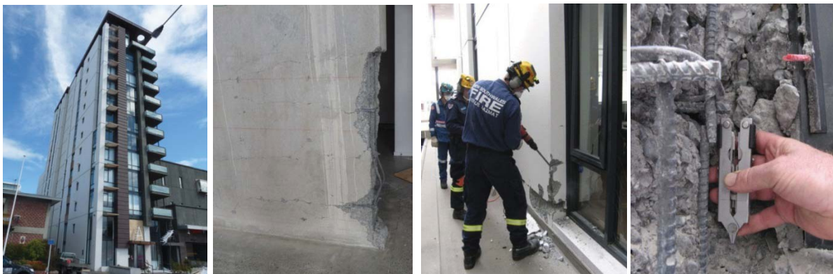
(a) Overall view (b) Wall damage (a) Concrete removal (b) Fractured bar
