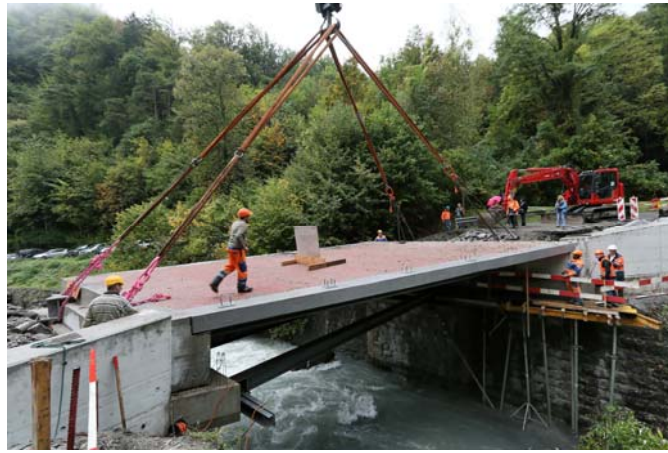
Figure 3.1: Installation of Avançon Bridge in Bex, Switzerland, 2012, semi-integrated balsa-GFRP sandwich deck adhesively bonded to steel main girders
