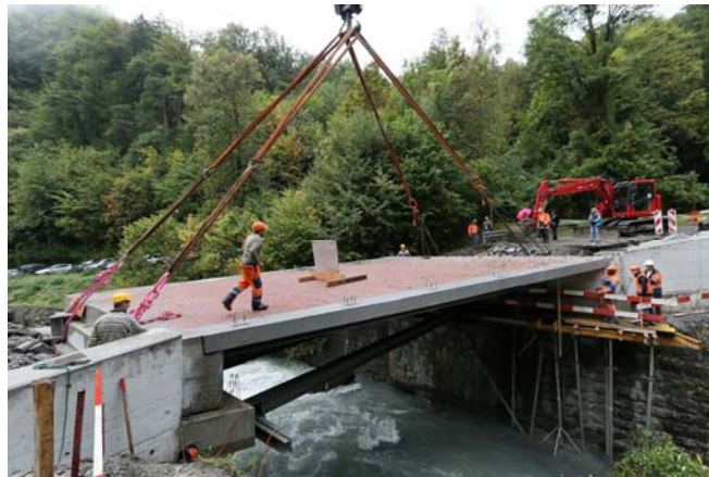
Figure 1.5: Installation of Avançon Bridge in Bex, Switzerland, 2012, semi-integrated balsa-GFRP sandwich deck adhesively bonded to steel main girders [30]
