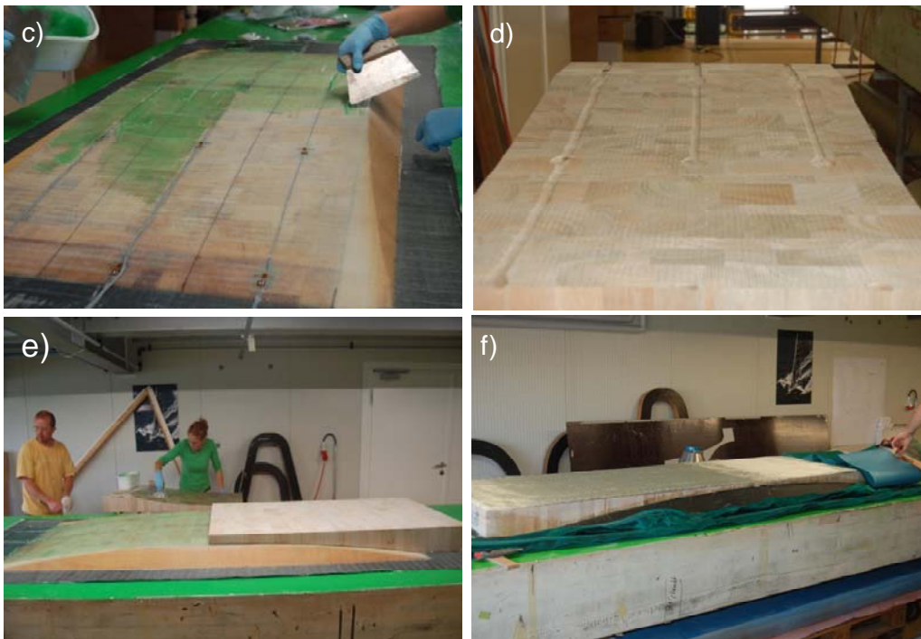
Figure B.2 (c) strain gauge installation and adhesive application on GFRP arch (A-G panel), (d) grooves for strain gauges in upper high-density balsa (SB150), (e) placing of upper high-density balsa and (f) laying-up of upper face sheet,
