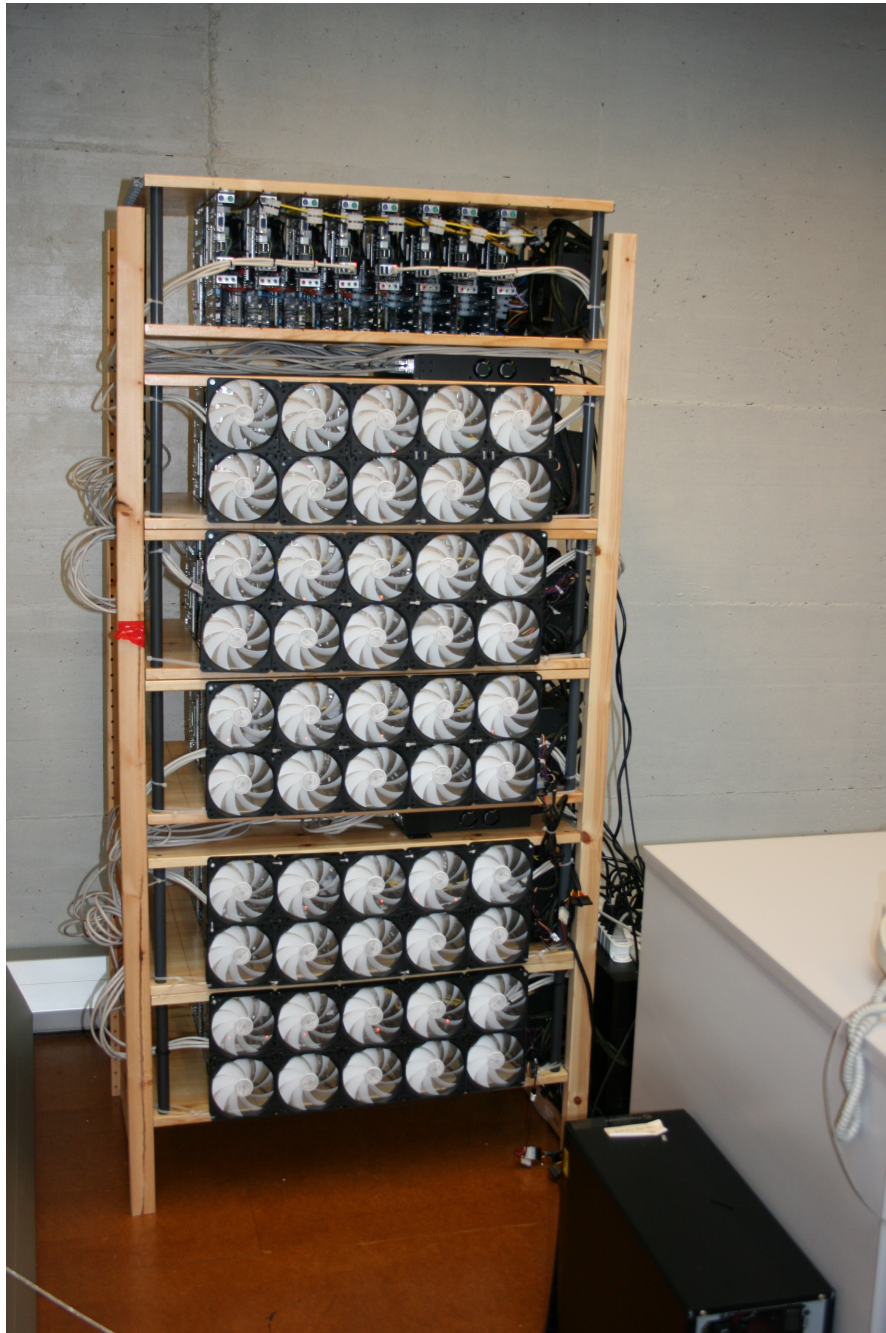
Figure C.1 – Front view of the cluster. The fans of the top shelf have been removed showing the motherboards stacked vertically in two rows such that each shelf carries 16 nodes powered by two power supplies.
