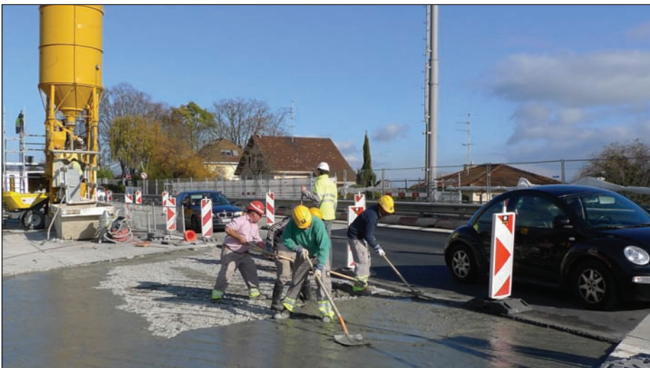
Fig. 9: Rehabilitation of a bridge deck of an underpass with UHPFRC: slope 5%, average external temperature of 5°C
