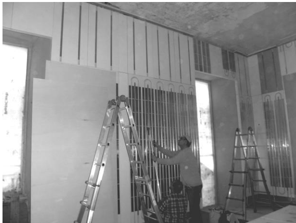
Figure 3: Insulating/radiant panels on the wall of the pilot room
