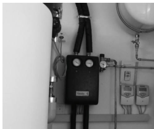
Figure 3: Photo of the storage, pump and controllers of a test system. Source: Egon AG
