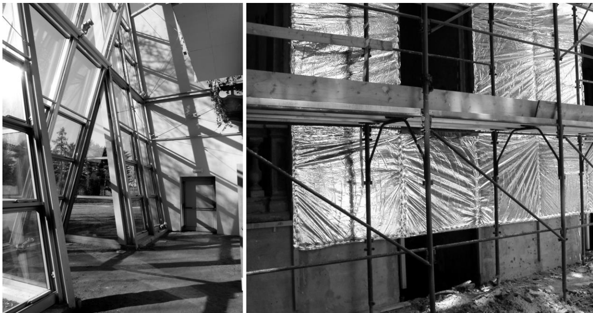
Figure 4: View of the greenhouse (left) and thin insulation used in the retrofitting (right).
