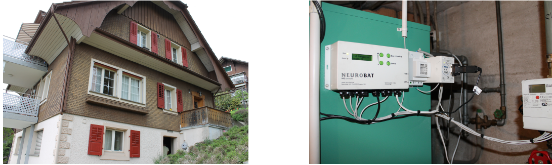
Figure 1: Left: the Ruswil test site. Right: the NIQ installed in Ruswil.
