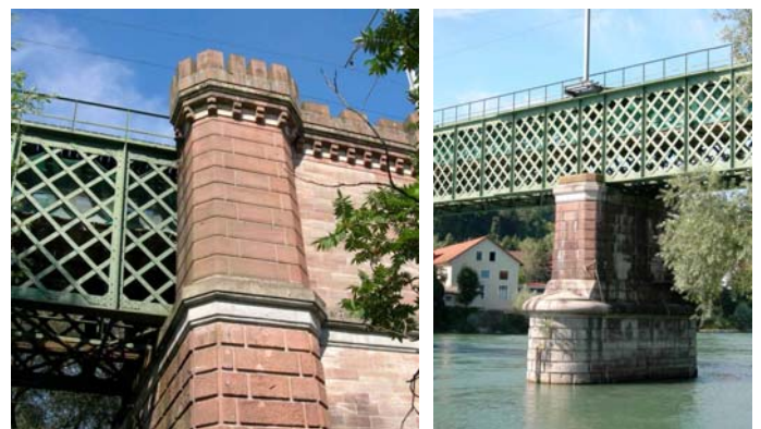
Figure 2. Details showing the interrelation between the wrought iron lattice girder and natural stone pier and abutment.
