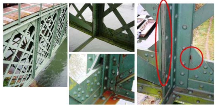
Figure 4. Condition of the corrosion protection coating.
