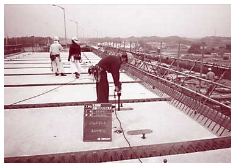
Fig. 1.4: In situ welding of shear studs inside the pockets of prefabricated deck [Japan Highway administration]
