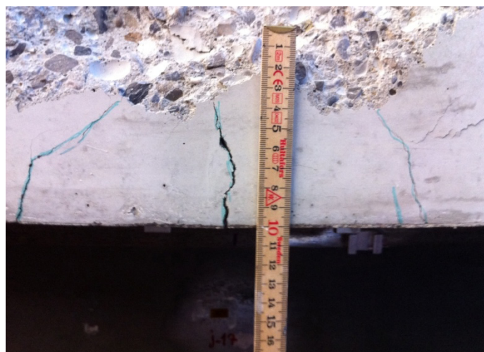
Fig. 4.22: Tensile cracking on the lower part of the reinforced concrete of the composite beam for the section with ultimate moment
