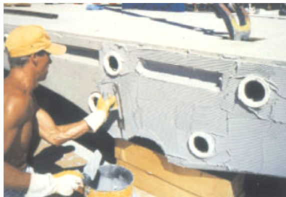
Fig.1.6: Trowel application of the adhering joint to prefabricated deck slab segments with sealing rings for the cable troughs [Dauner 2006]
