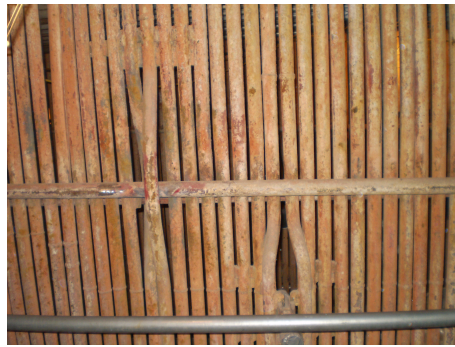
Figure 1.3: Example of boiler tubes of 50 mm diameter.
