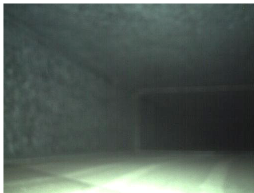
Figure 3.4: Camera view of the Cy-mag 3D II in an air duct.
