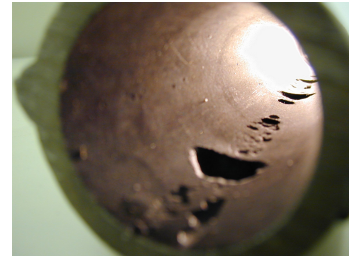
(c) Tube pitting (source: Consultant Surveyor)
