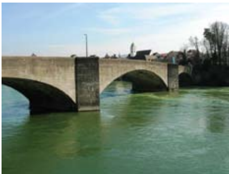
Figure 1. Historical concrete bridge over the Rhine river at Rheinfelden, designed and built by Robert Maillart in 1912.
