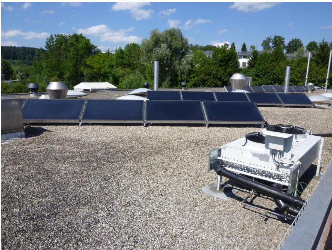
Figure 2: Photo of the flat plate collector field (back) and the heat rejection cooler (front right).
