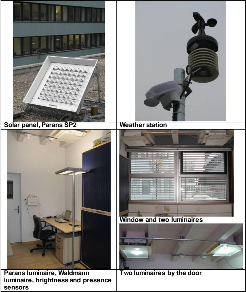
Figure 2: The Clear-up project test office at Siemens HVAC Lab in Zug. The components and layout for the equipment steered by an automatic building management system.
