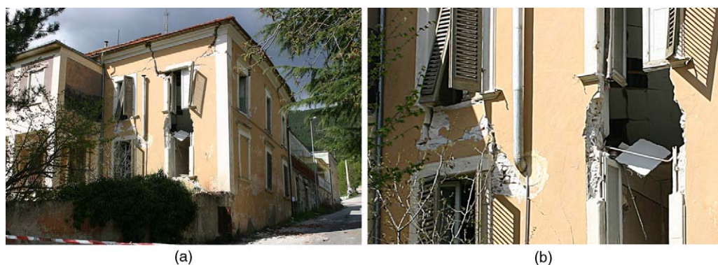
Figure 2. Flexural failure of spandrels in an old URM building after the L'Aquila earthquake on 6 April 2009: (a) Entire building and (b) detail of a spandrel.
