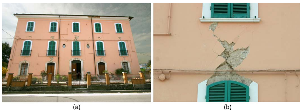
Figure 1. Shear failure of spandrels with shallow masonry arches in an old URM building after the L'Aquila earthquake on 6 April 2009: (a) Entire building and (b) detail of a spandrel.
