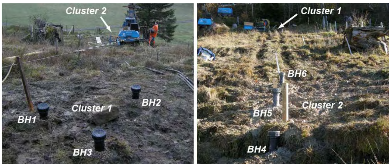
Figure C.1: Cluster 1 with boreholes 1 - 3 and Cluster 2 with boreholes 4 - 6. Cluster 2 is located 20 m downslope of cluster 1. Borehole 6 is equipped with 2 piezometers. All others are equipped with 1 piezometer.
