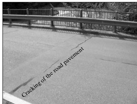
Fig. 8: Cracking of the road pavement at the connection between the transition slab and the bridge deck, semi-integral bridge of 68 m length built in 1986 in Reichenau/CH 8
